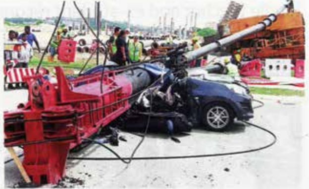
Horrific end: The collapsed piling machine which killed Abd Rahim and his wife Nurhayati at Persiaran Astana in Meru, Klang.
